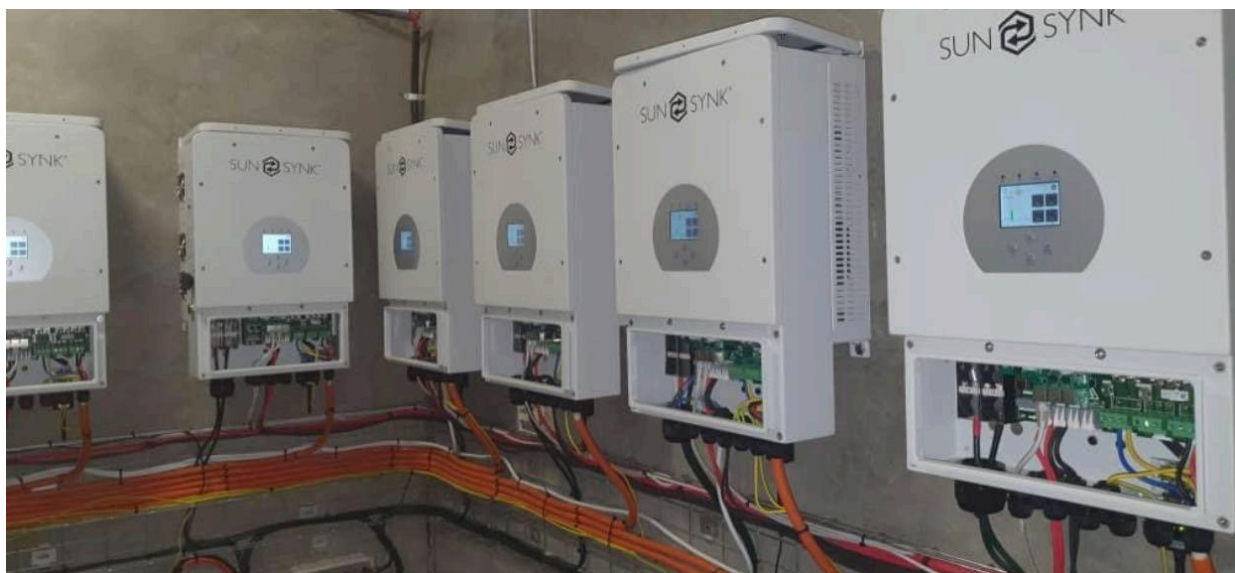
Figure 55 - Sunsynk inverters paralleled.
