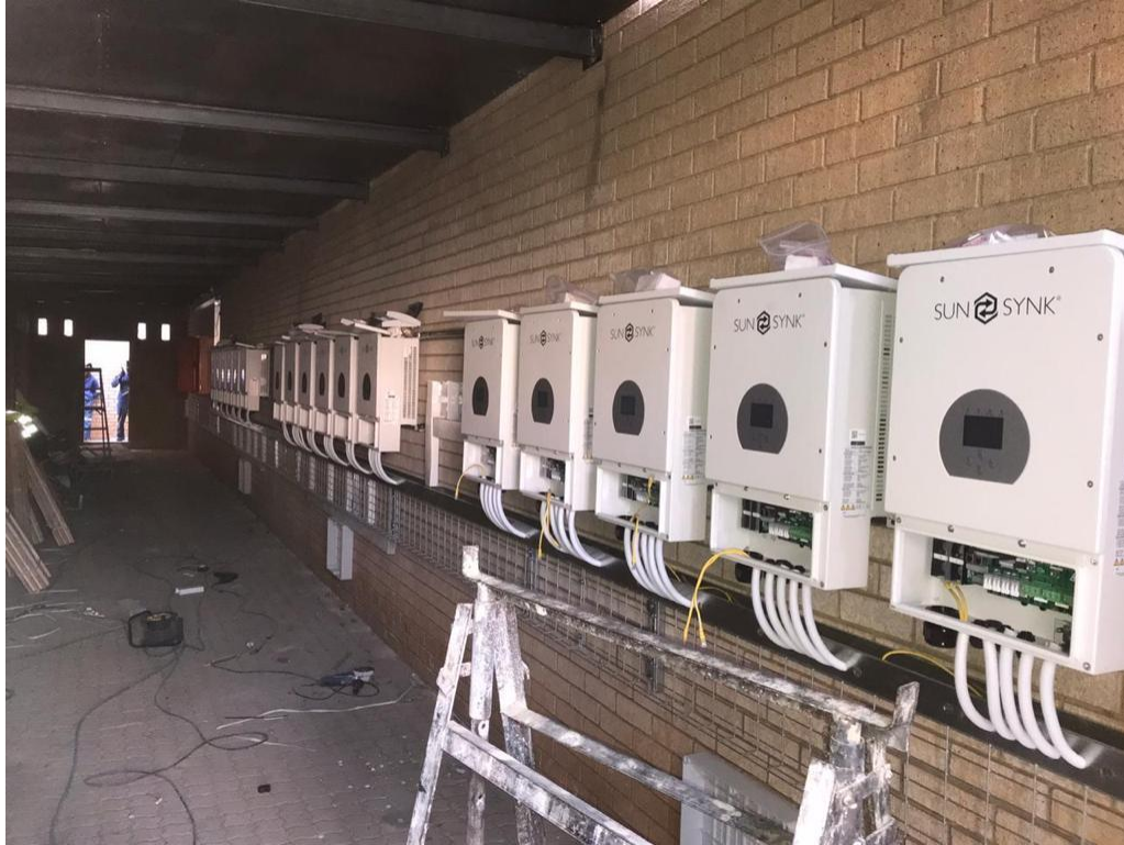
Figure 51 - Installation with many inverters.
