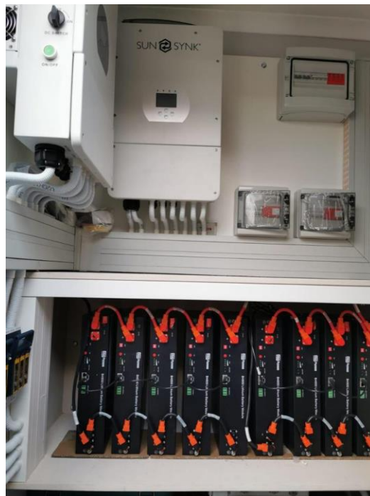
Figure 16 - Inverters with appropriate battery connections.
